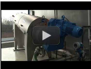
Video: HUBER Screw Press Q-PRESS@ - here at a municipal WWTP https://www.youtube.com/watch?v=5VsPNKbkJyA
