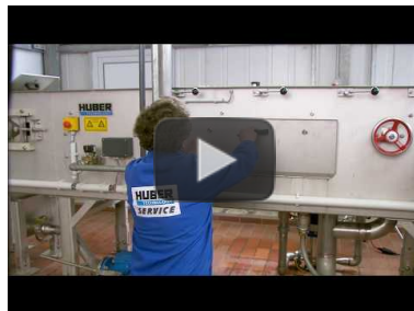
Video: HUBER Belt Thickener DrainBelt - here at a municipal WWTP https://www.youtube.com/watch?v=6pcHf8aJpqQ
