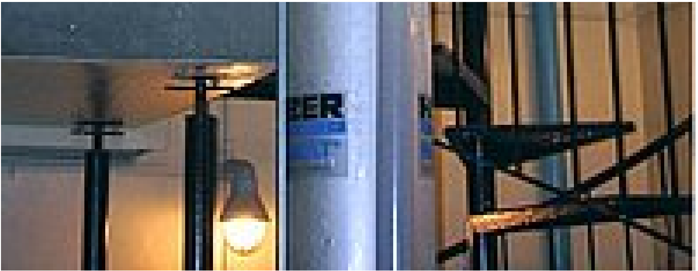
Vertical screenings transport tube of the RoK 4
