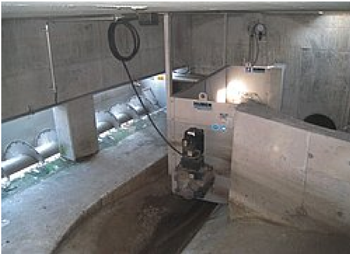
Stormwater overflow tank at Kappern: Storm Screen RoK1 on the left, Storm Screen RoK2 in the middle on top of the sewer towards the WWTP
