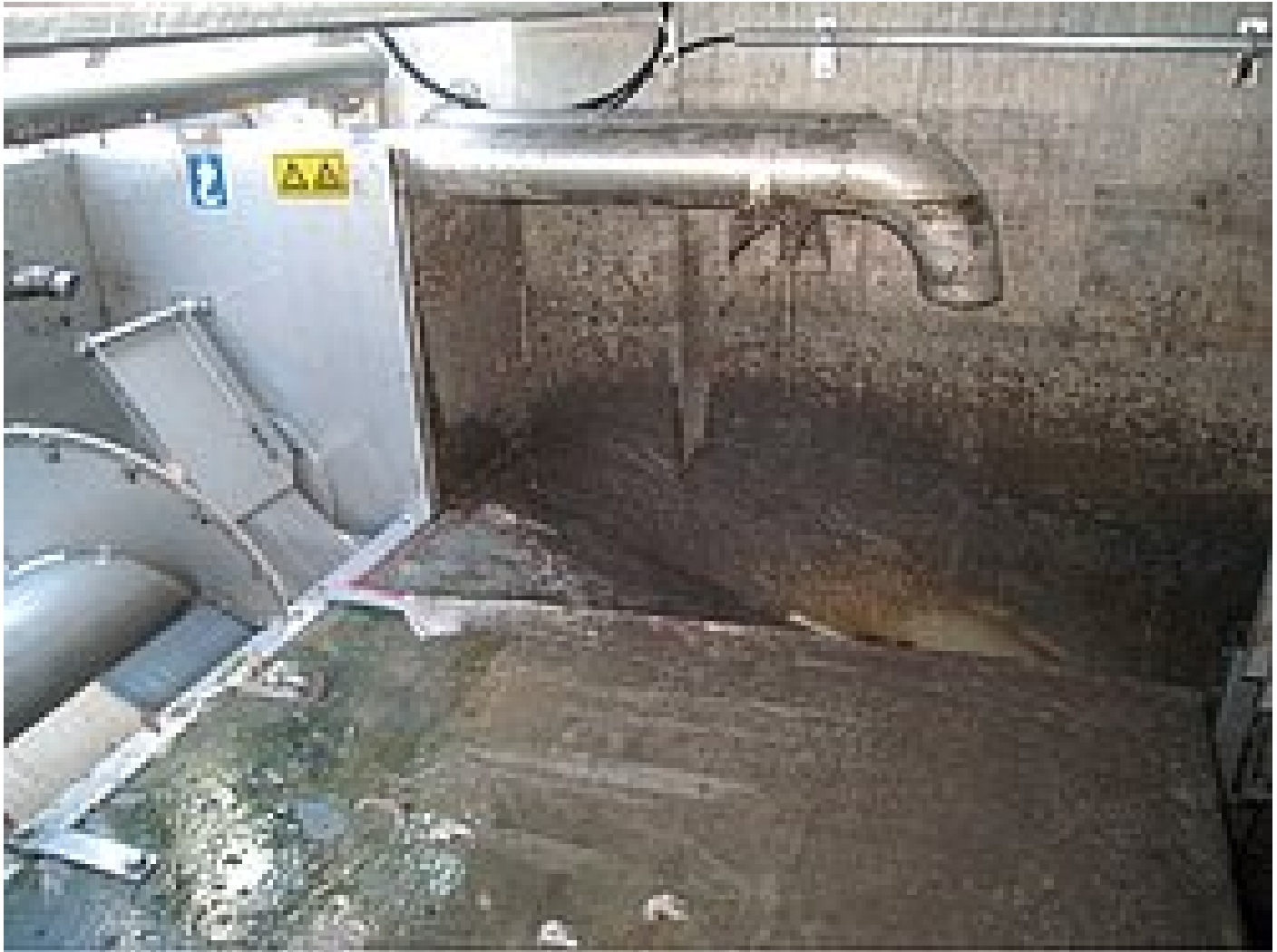
Screening laundry channel built into the berm, washing system at the left, discharge line on top
