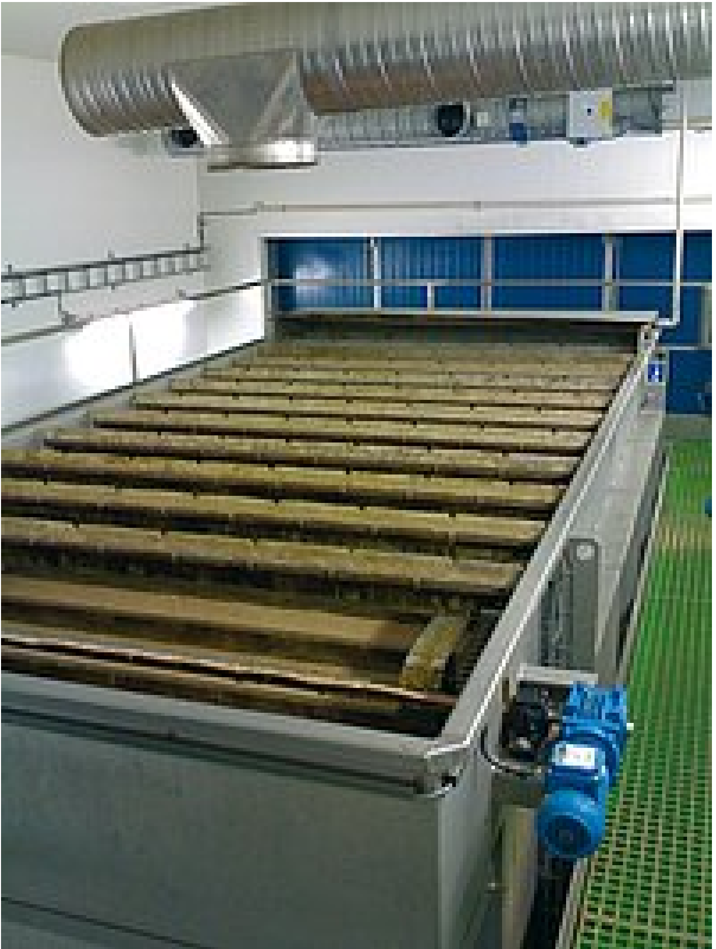
HUBER HDF 10 at the slaughterhouse in Ringsaker, Norway
