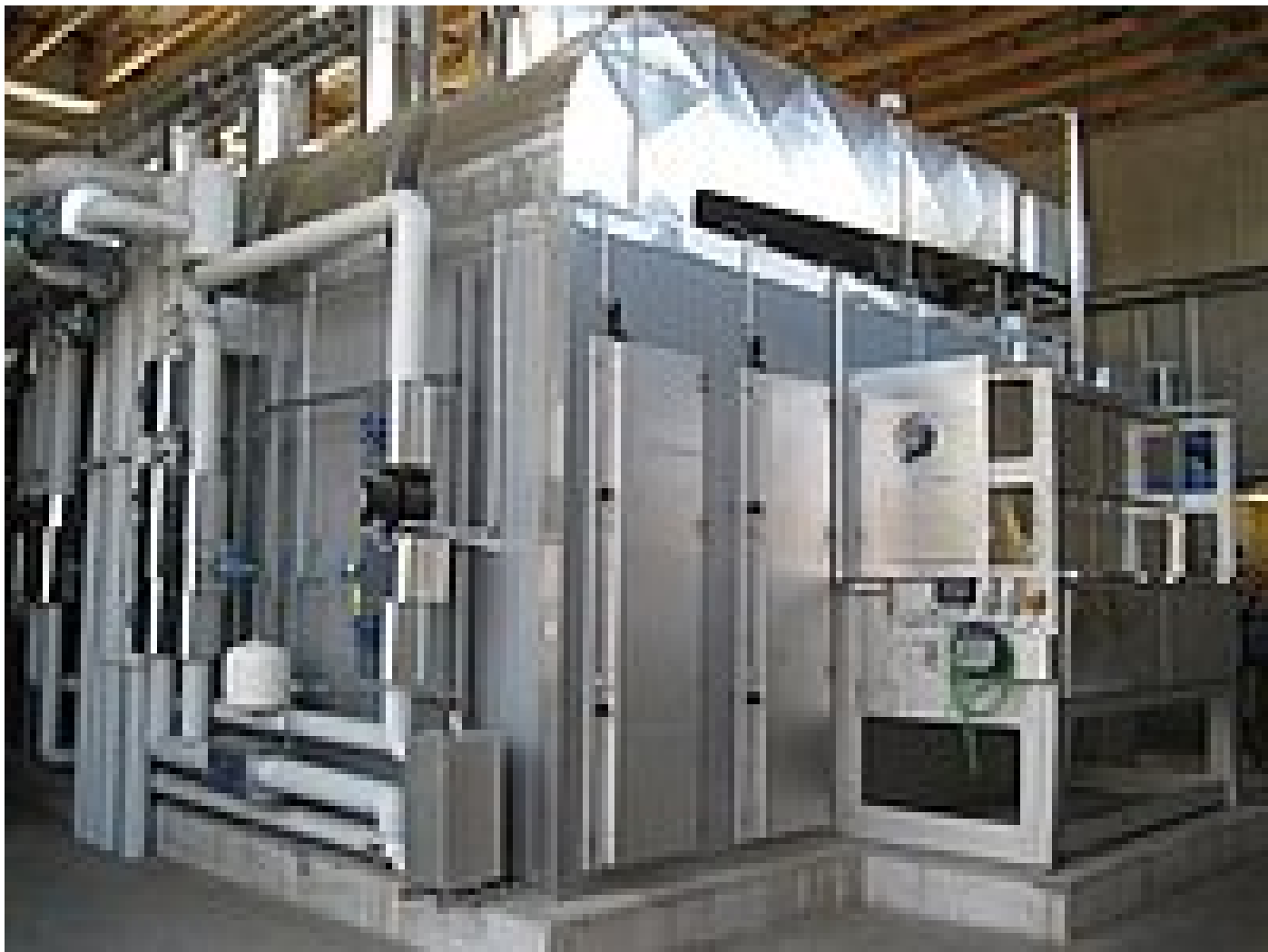
Fully isolated two-stage belt dryer installed on WWTP Balingen
