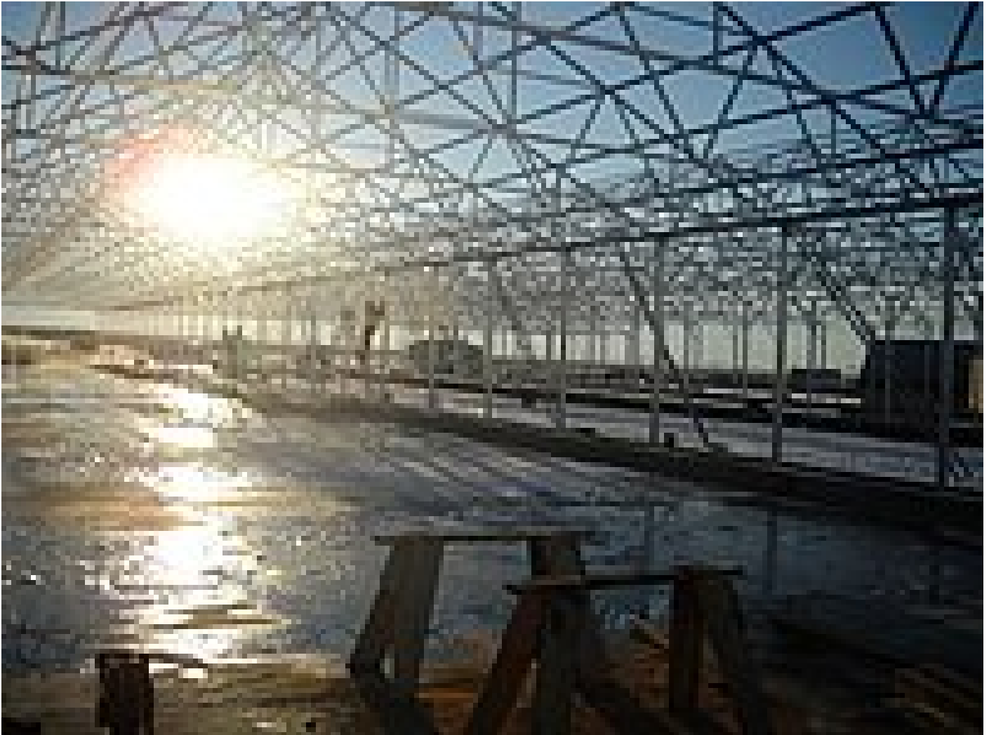
Solar dryer under construction at Utah – a reasonable solution even in climate zones with cold winters
