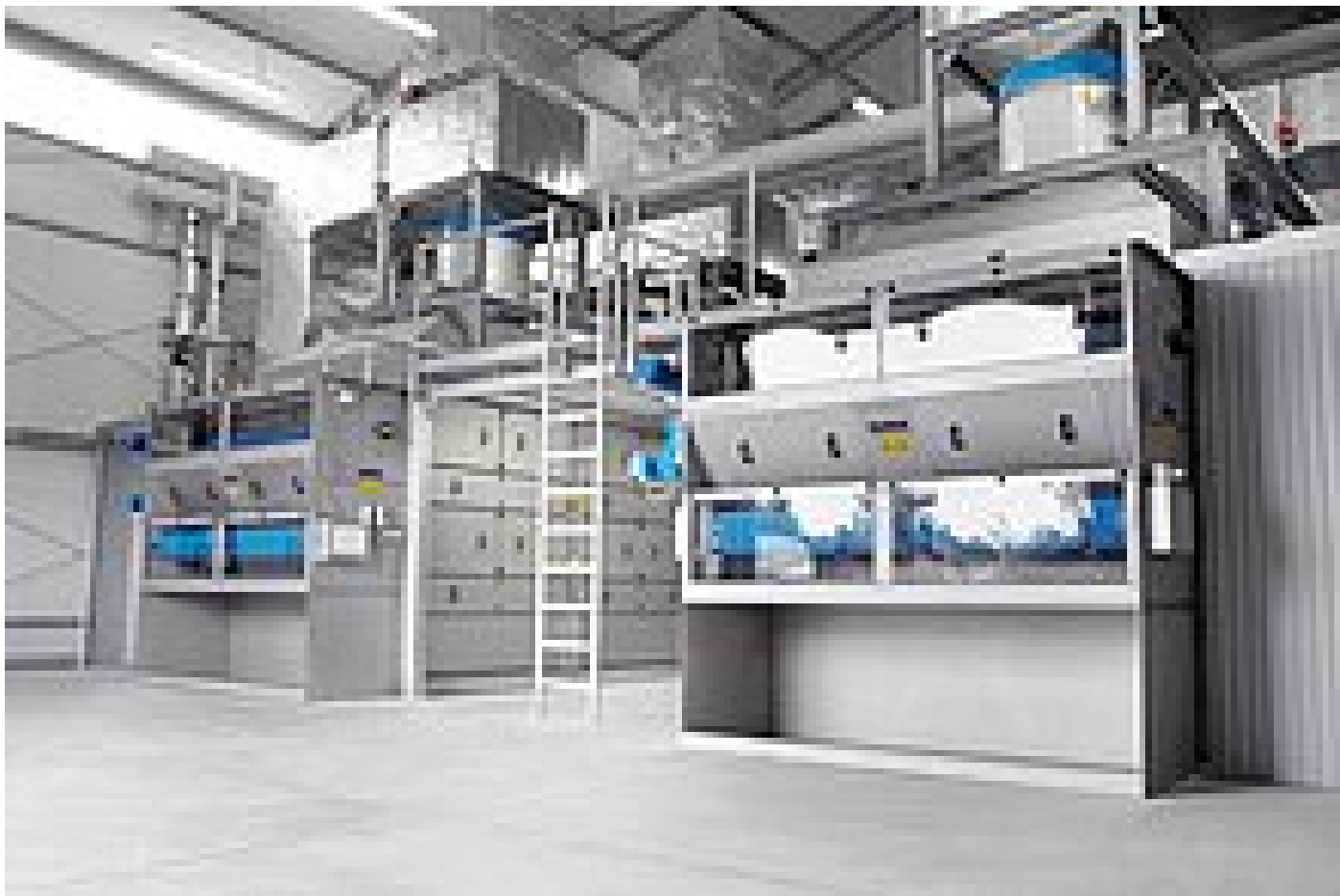
HUBER Sewage sludge drying plant on STP Ingolstadt
