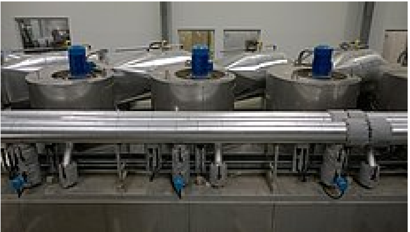
Hot water supply and ventilators of the sludge dryer with V4A insulation
