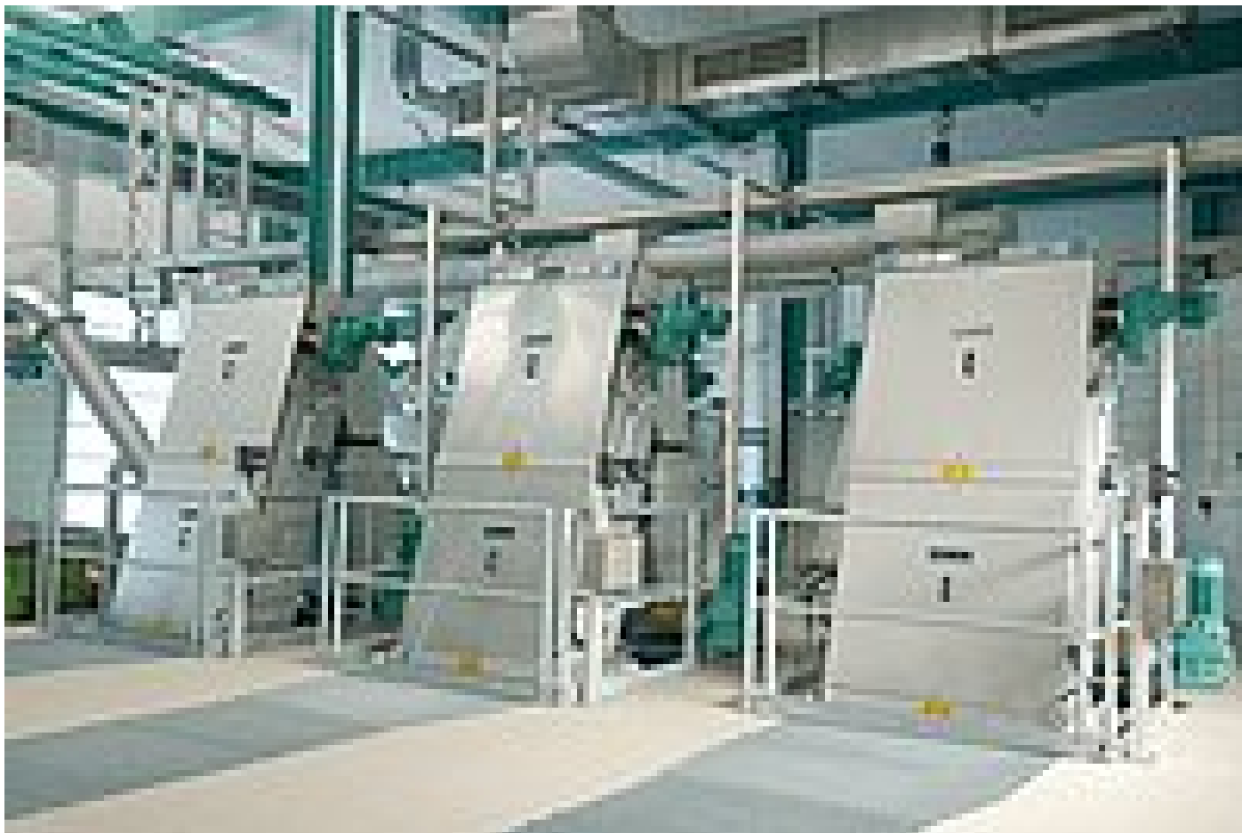
These RakeMax® screens at the WWTP Zwickau are exemplary for their combination of sturdiness and performance
