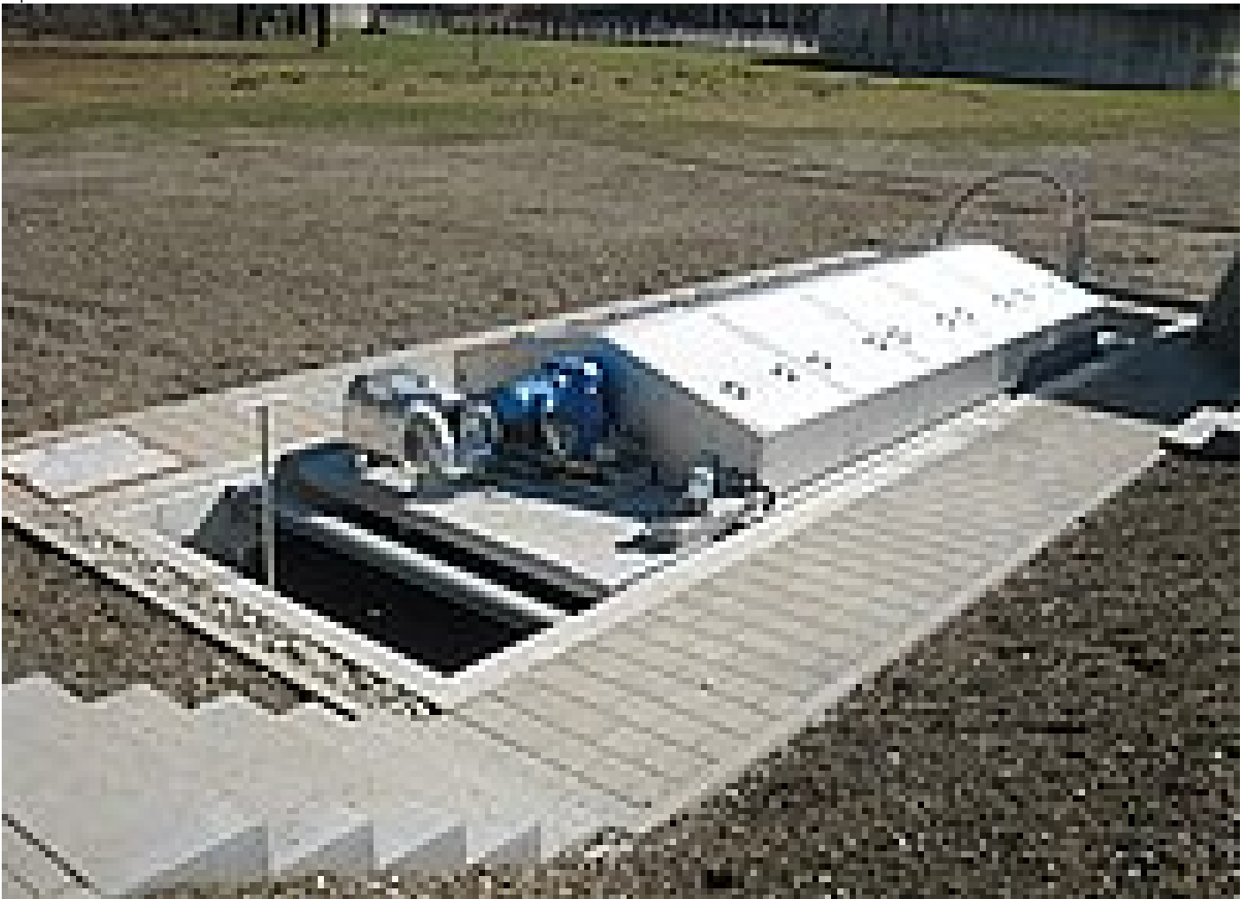
RoDisc® Rotary Mesh Screen installed on WWTP Altötting
