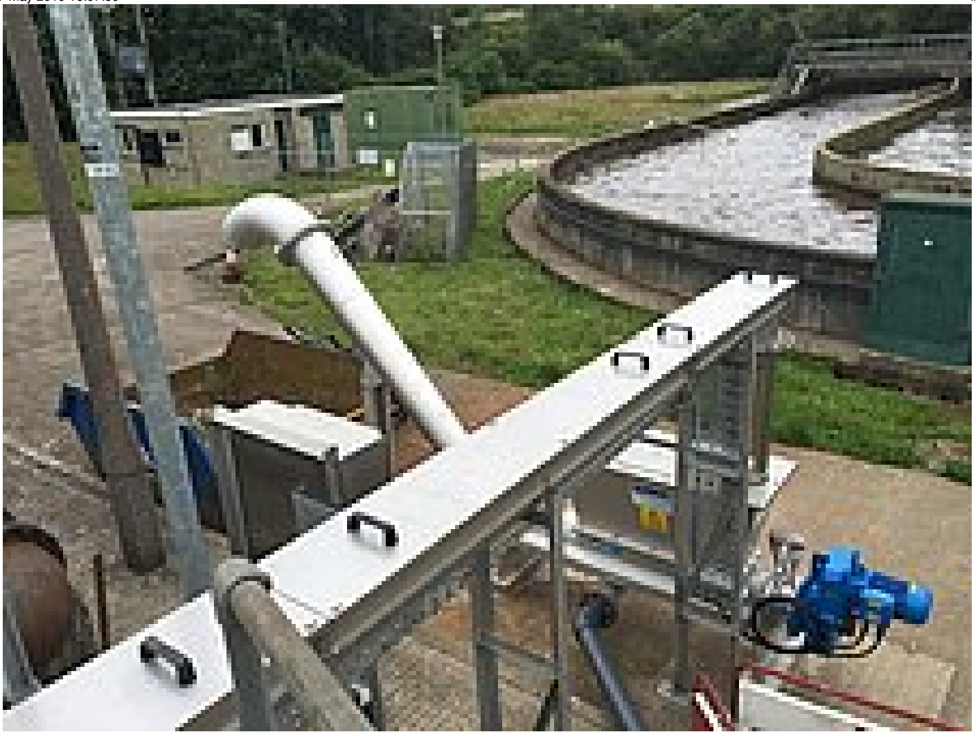
Launder Channel feeding the Wash Press
