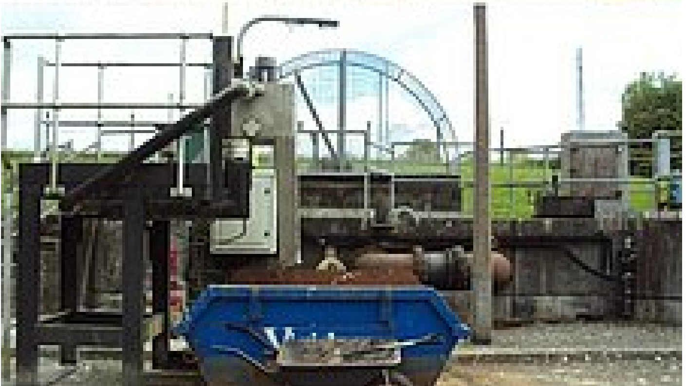
The old equipment installed was at the end of its asset life and constantly failing
