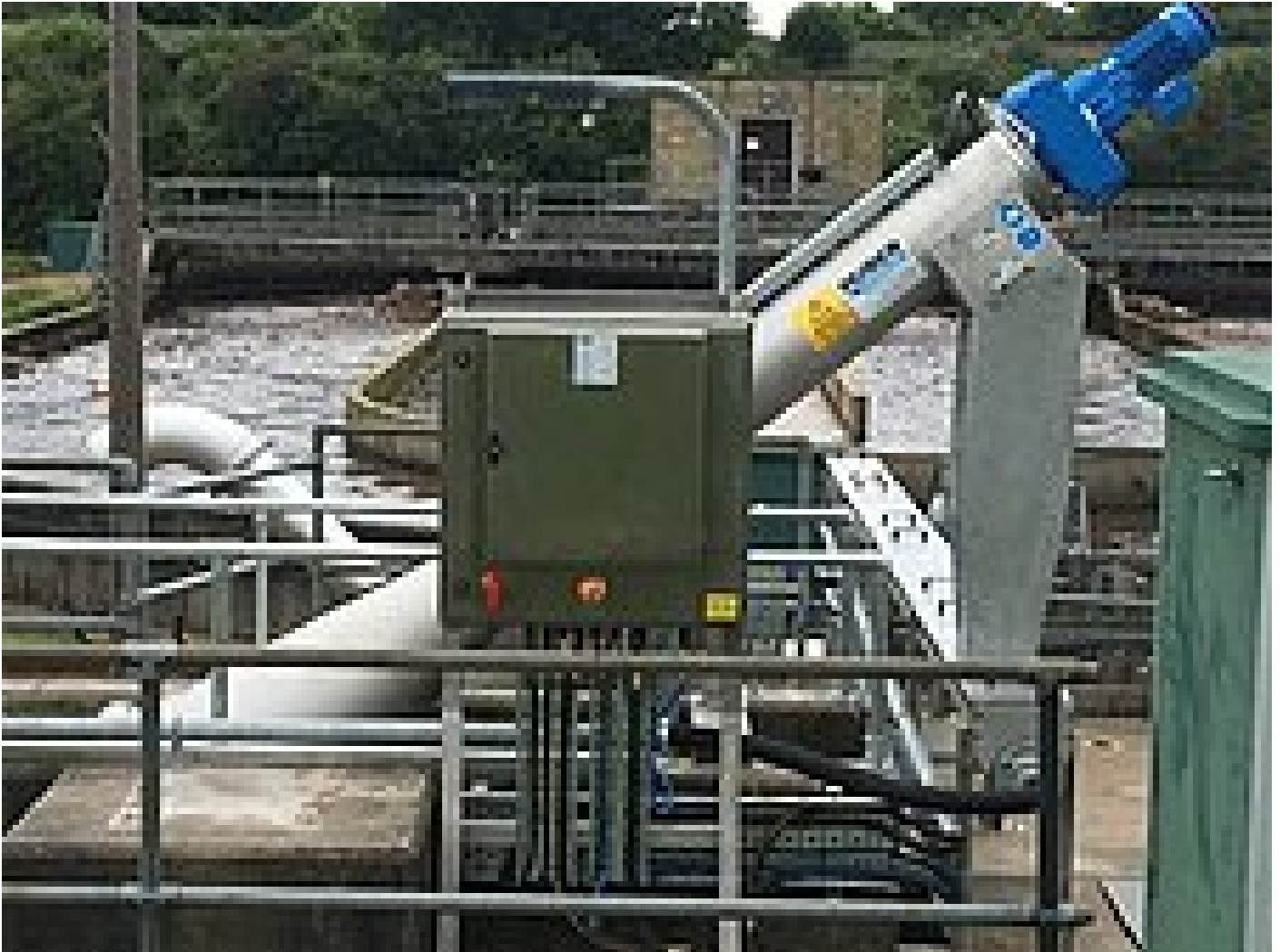
HUBER Micro Strainer ROTAMAT® Ro9 installed at Charfield STW
