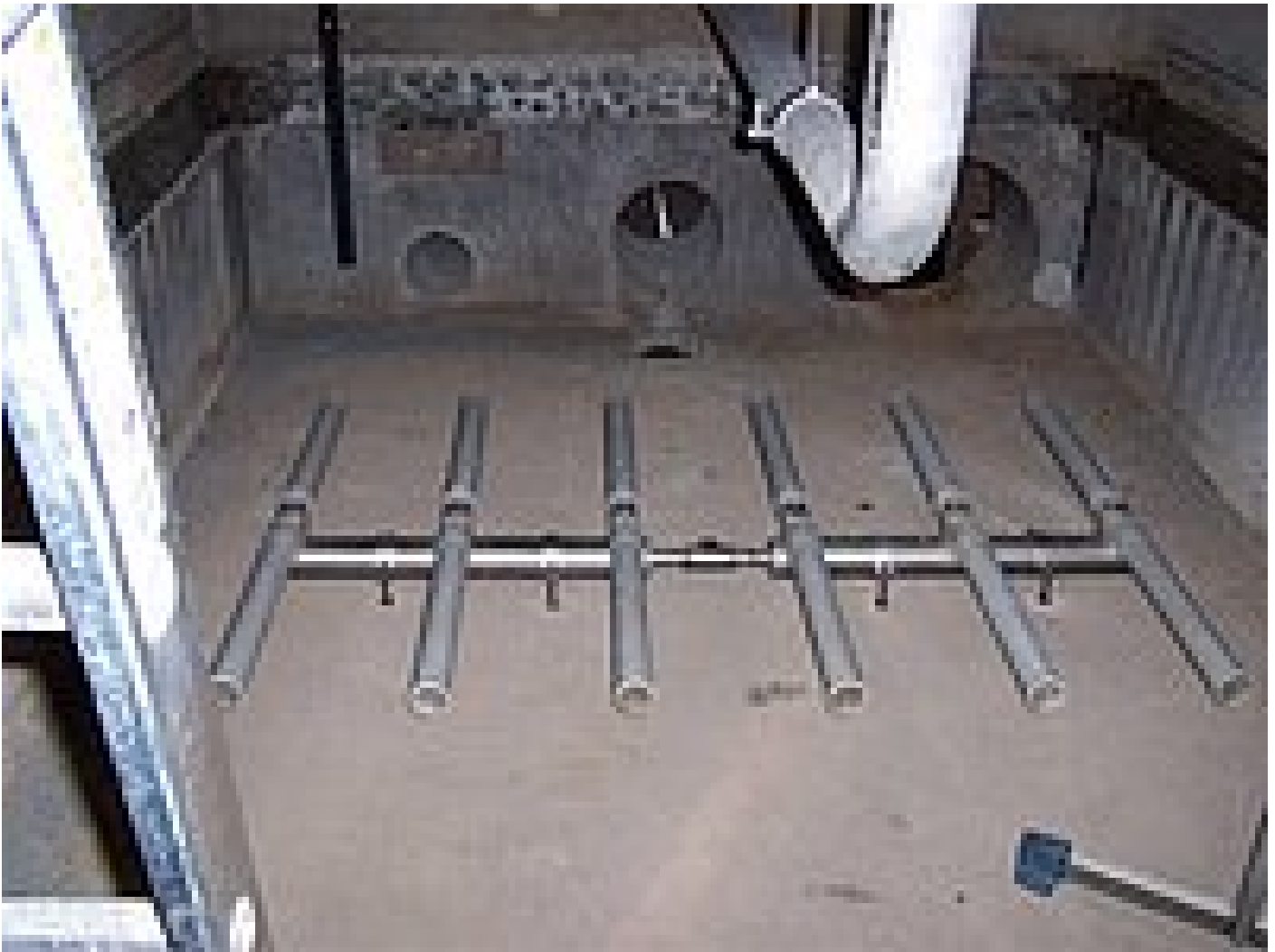
Aeration by fine bubbles
