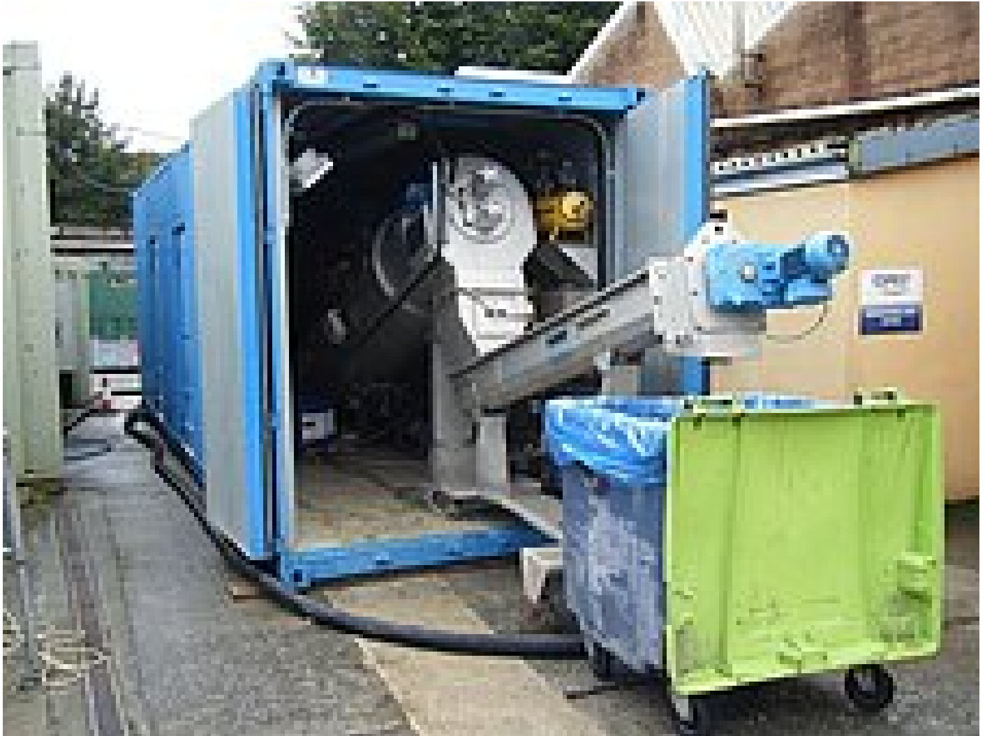
ROTAMAT® RoS3.2 industrial trial unit at the effluent plant of Premier Foods Ltd., Lifton
