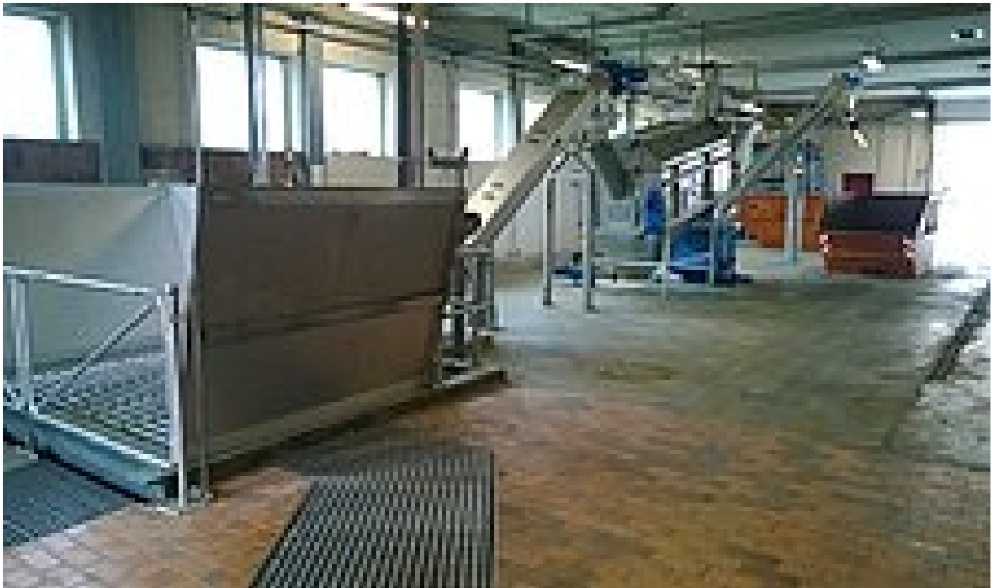
Grit acceptance system RoSF5VW on STP Koblenz
