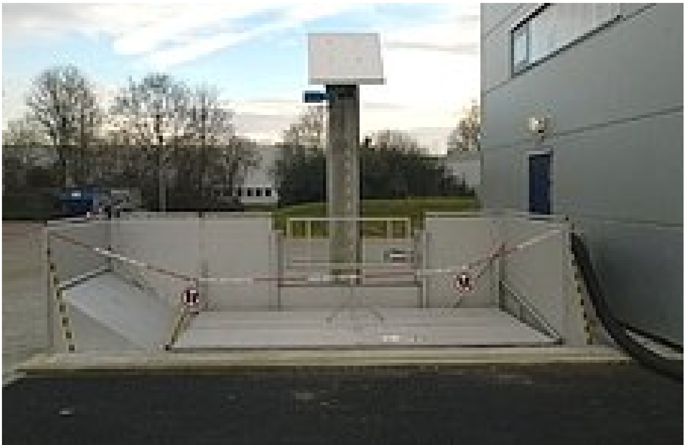
Grit treatment system RoSF5HW with automatic covering of the acceptance tank on STP Frankfurt Niederrad
