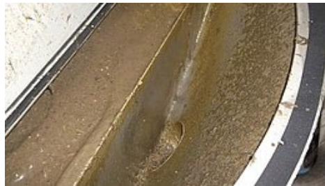
... of removed grit and returned to the flow
