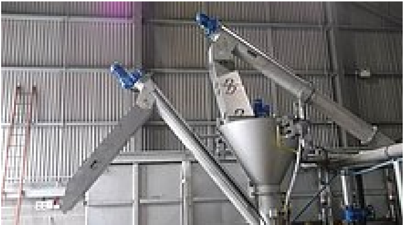
Grit washer was elevated so that the overflow drained back to the grit trap
