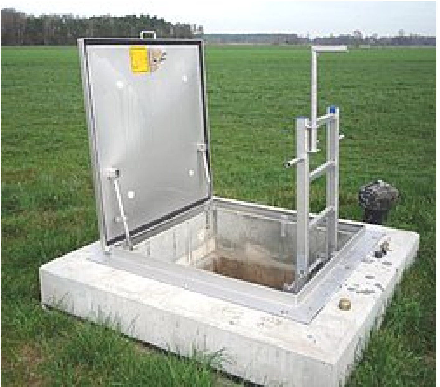
Safe equipment: manhole covers, safety access ladder and entrance aid
