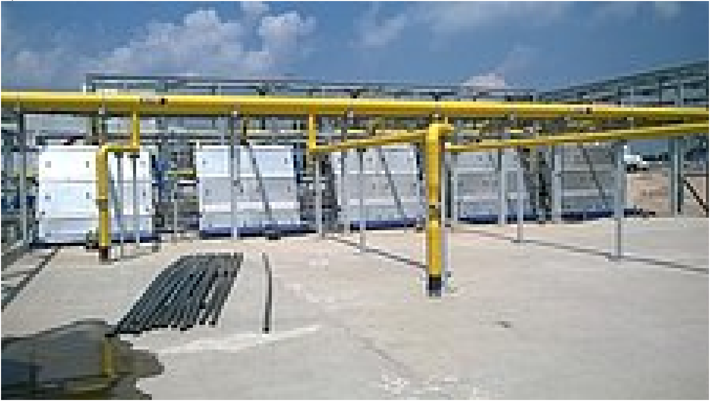
WWTP Atotonilco, the first of two coarse screen lines with 5 big HUBER RakeMax® screens, with direct discharge into a HUBER Launder Channel HLC with a length of 30m
