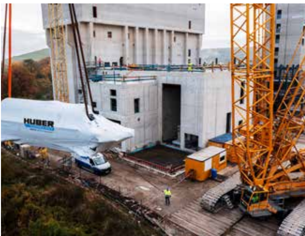
A disc dryer is lifted into place with the help of a heavy-duty crane.
