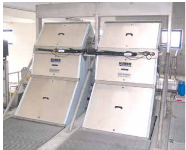
Two HUBER Fine Screen STEP SCREEN® SSF units installed in parallel channels.
