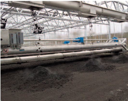
Automated sludge feeding
