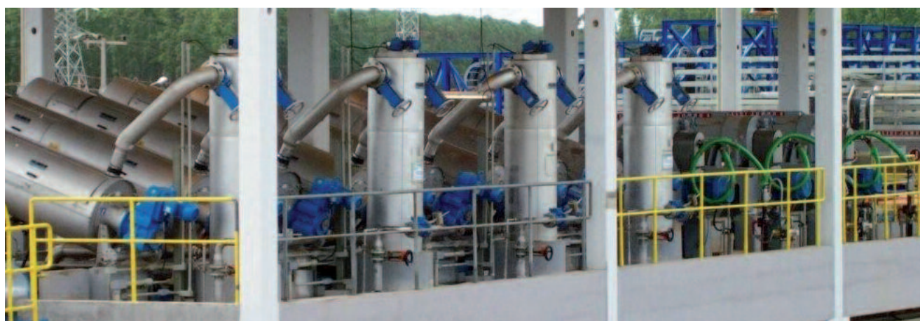
4 x 2 ROTAMAT® Screw Press RoS 3 units installed in parallel (Brazil)
