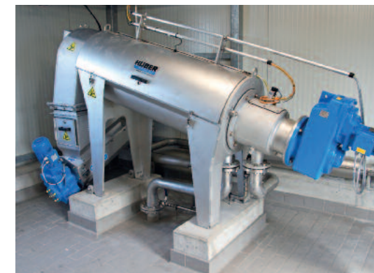
The sludge dewatering unit directly before sludge drying
