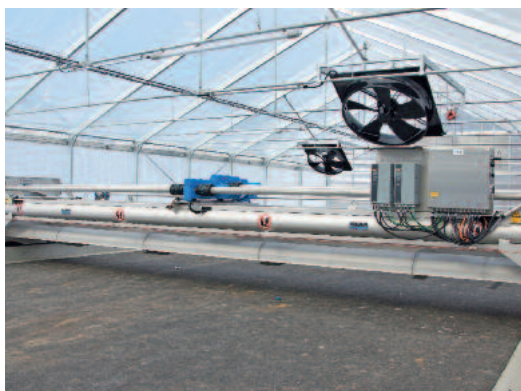
The solar sewage sludge drying plant shortly before commissioning
