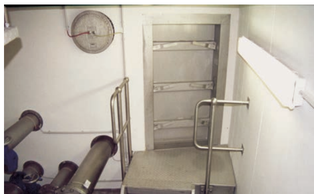
Access to water chamber
