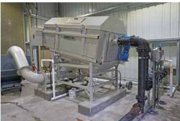
HUBER Sludge Acceptance Plant RoFAS with metering system for pH and conductivity measurement.
