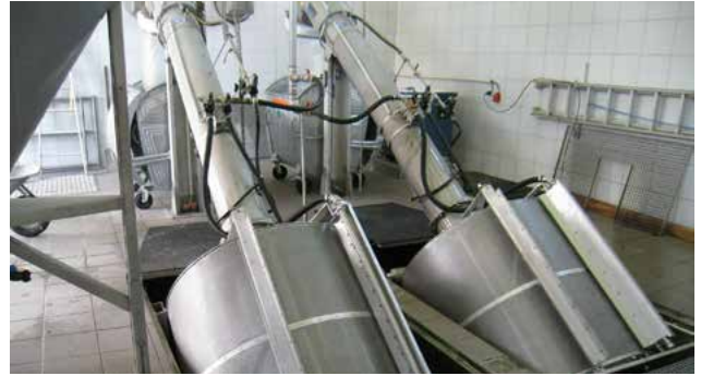
Low space requirement due to the use of two HUBER Rotary Drum Fine Screen ROTAMAT in the channel - size 1400.
