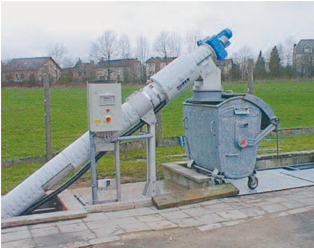
Outdoor installation of a HUBER Fine Screen ROTAMAT® Ro1 with frost-protection
