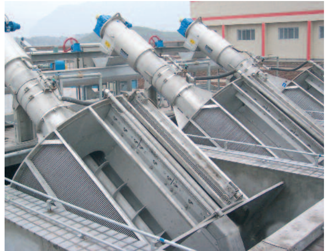
Several parallel HUBER Fine Screen ROTAMAT® Ro1 units installed in the channel
