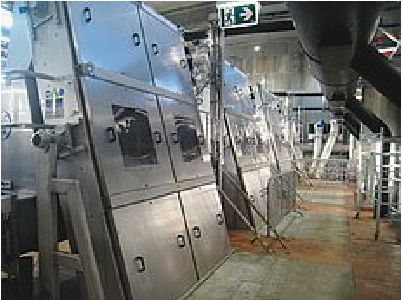
Most advanced technology: HUBER machines on STP Linz-Asten, the largest sewage treatment plant in Upper Austria
