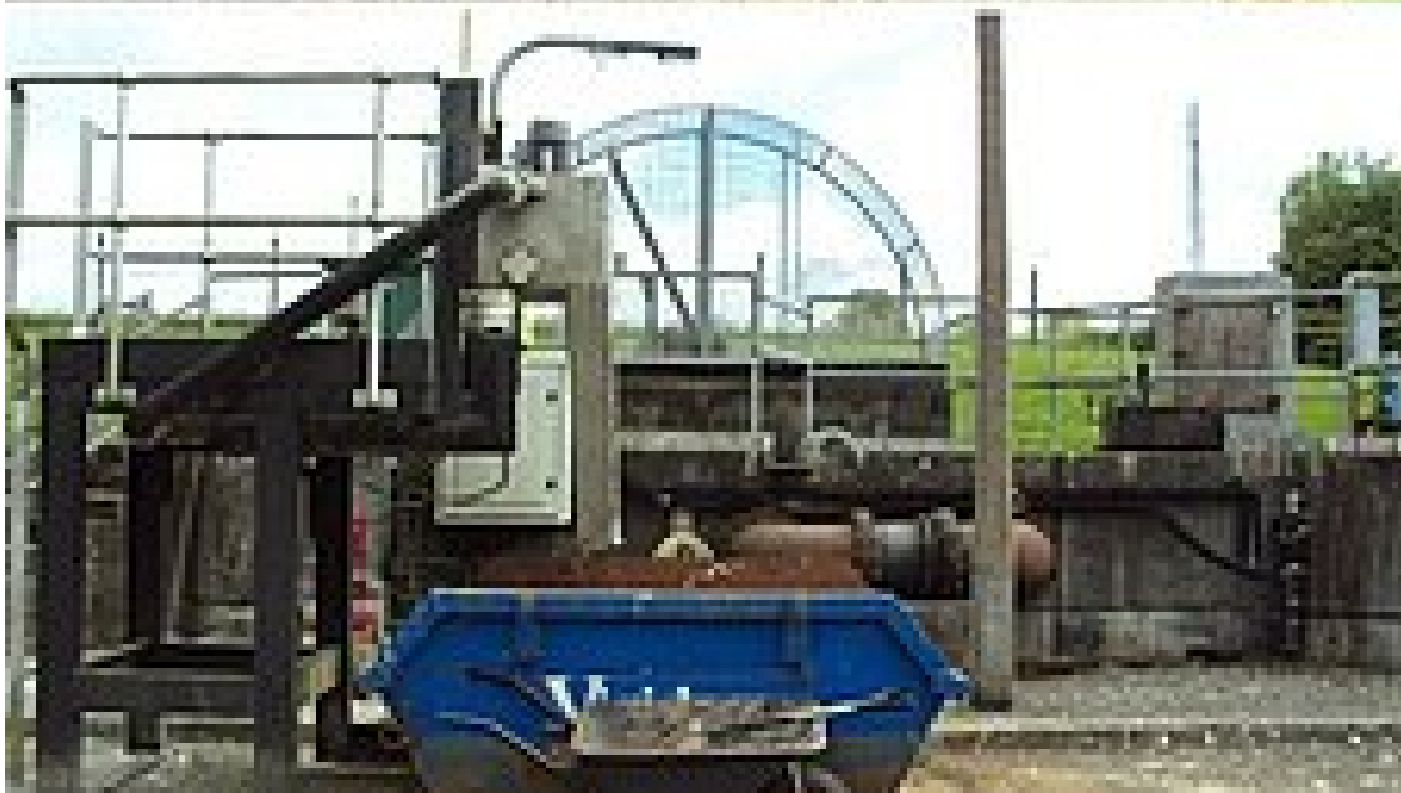
The old equipment installed was at the end of its asset life and constantly failing
