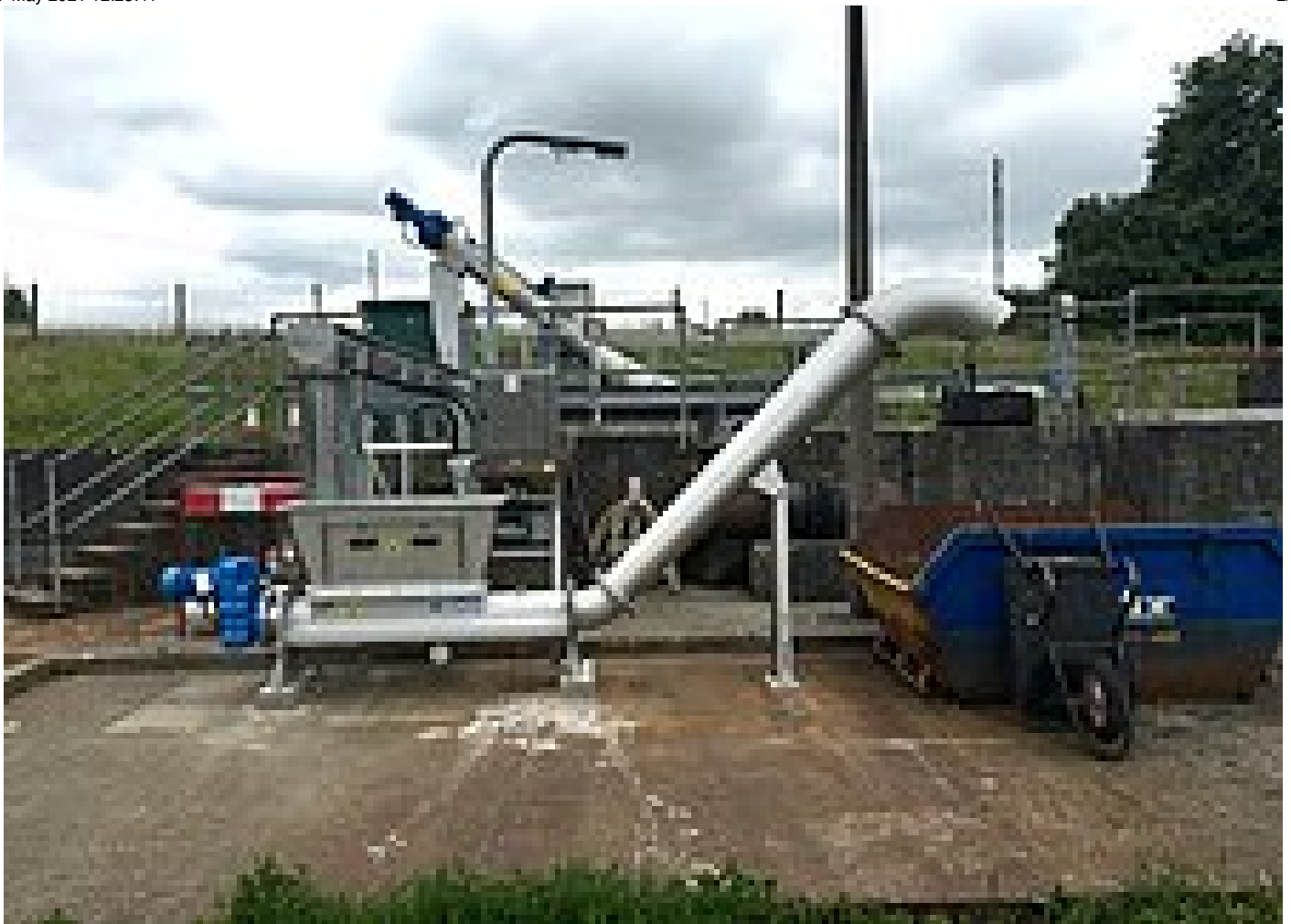
The complete HUBER installation with Wash Press WAP®/L in the foreground
