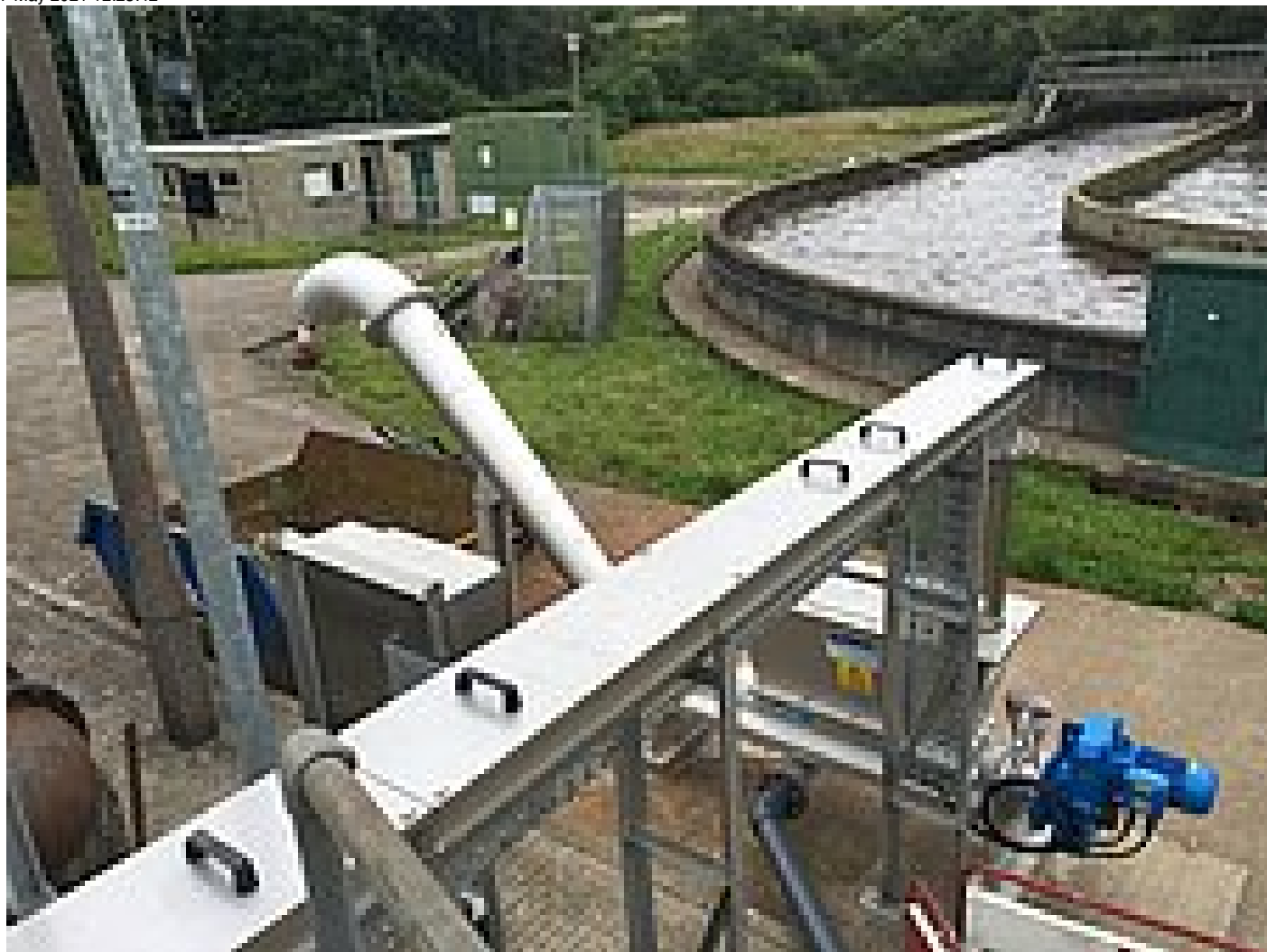
Launder Channel feeding the Wash Press
