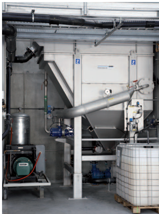
HUBER Dissolved Air Flotation Plant for process water treatment
