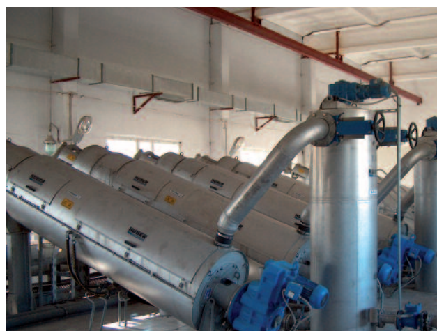
3 x 2 ROTAMAT® Screw Press RoS 3 units installed in parallel (Ukraine)
