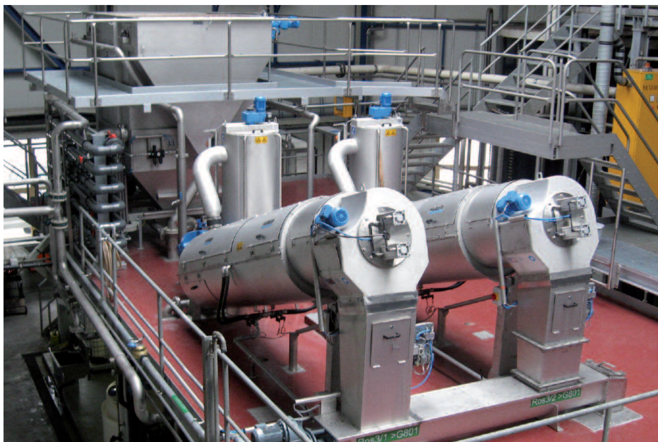
ROTAMAT® Screw Press RoS 3 units and HUBER Dissolved Air Flotation Plant HDF 5 with chemical treatment stage
