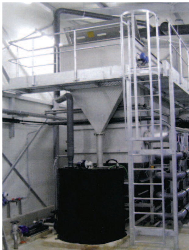
HUBER Dissolved Air Flotation Plant HDF 10 during start-up
