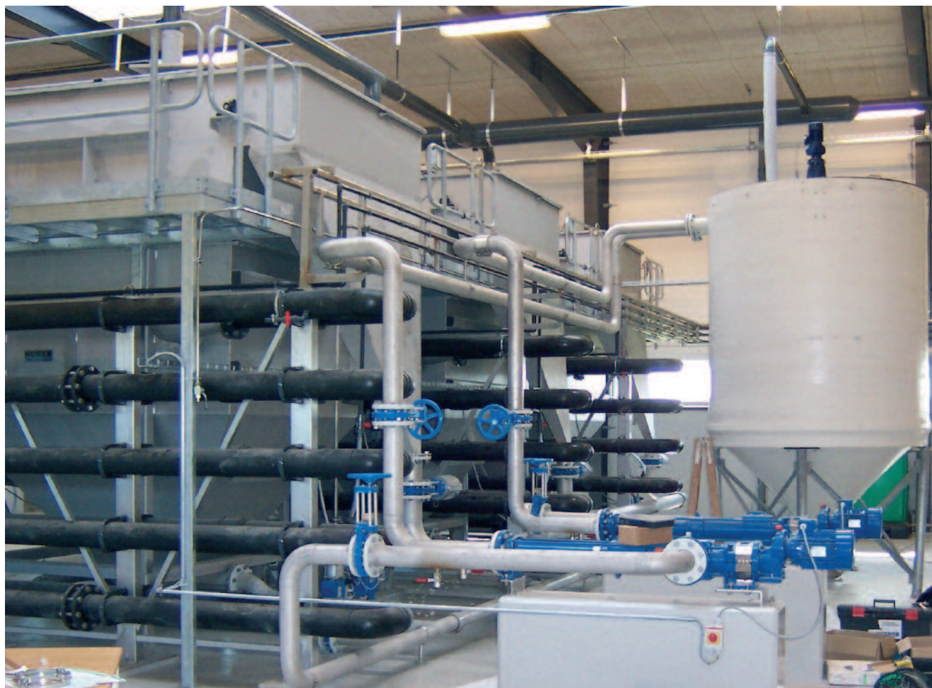
HUBER Dissolved Air Flotation Plant HDF 7 with chemical treatment stage and sludge tank
