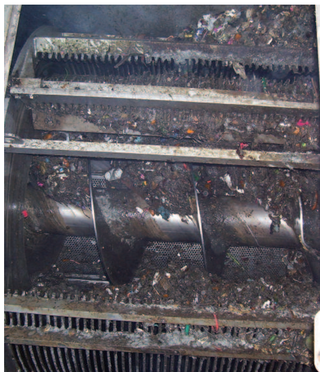
In the fine screening plant undissolved solids are removed from the organic suspension (approximately 5 - 15 % of the inflow)
