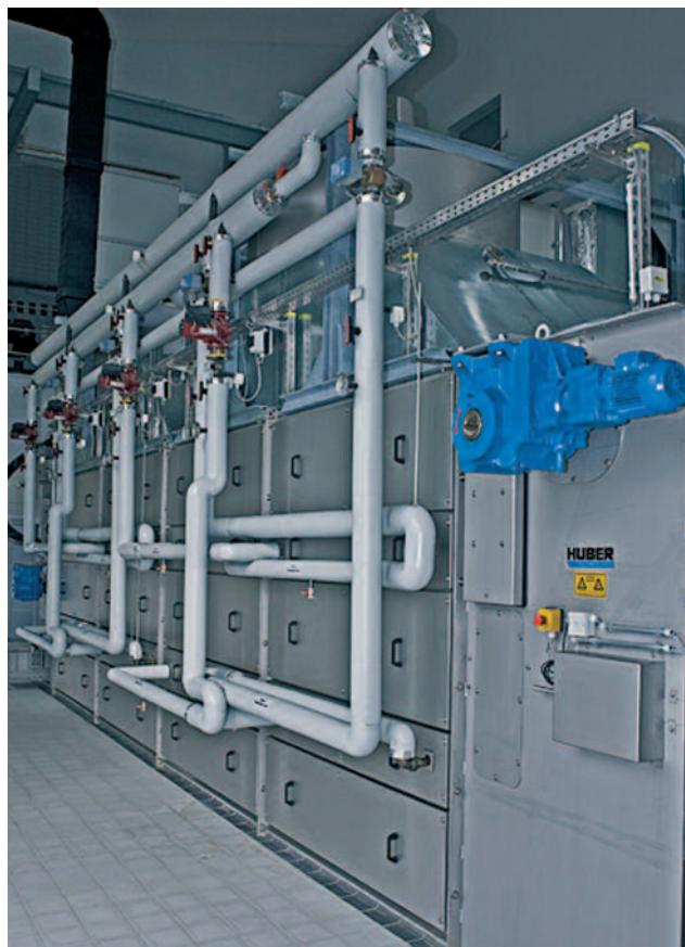
Biogas exhaust heat supply to a belt dryer
