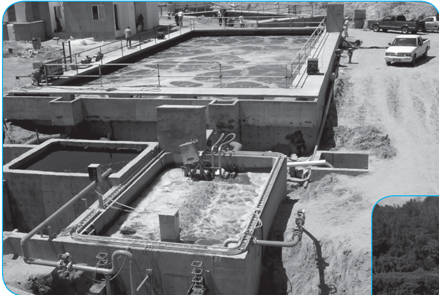
The 640,000 gallons per day MBR plant for a tourist resort in Los Cabos, Baha California, only took 8 months from preliminary design to final start-up of the membranes.
