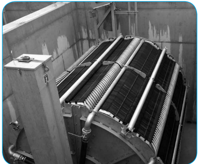
The Arenas de Iguña facility in Spain was the the first MBR plant to use Huber's VRM 30 unit.
