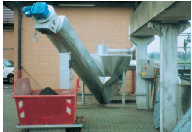
COANDA Grit Classifier installed subsequent to a grit channel
