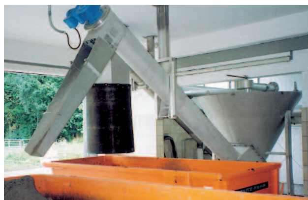
RoSF 3 COANDA Grit Classifier installation
