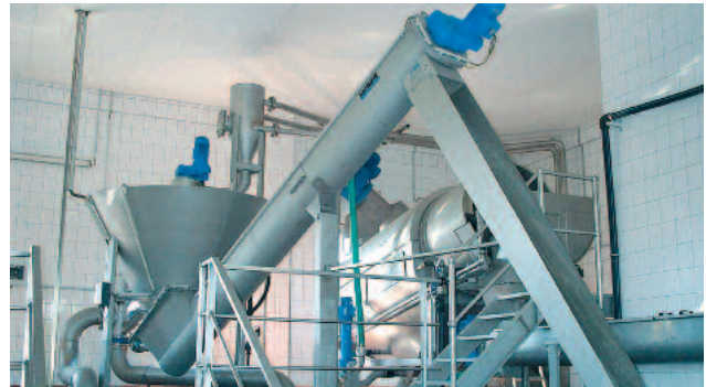
Wash Drum and Grit Washer installed in the customer's building
