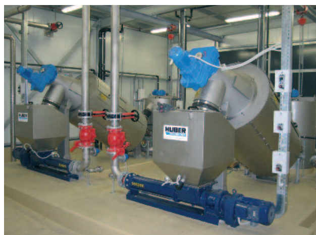
Two RoS 2 units for 80 m 3 /h
