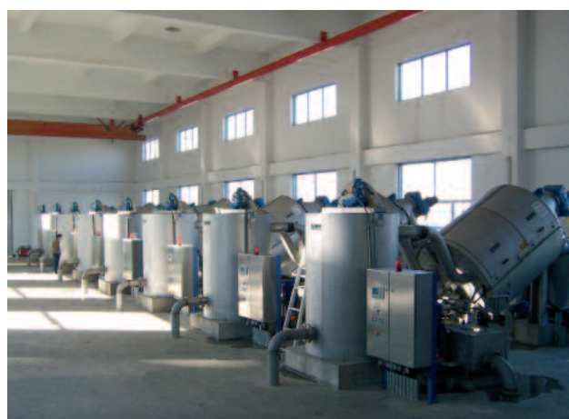
Several units installed in parallel to handle 600 m 3 /h
