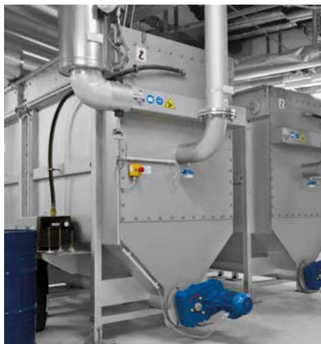
Municipal wastewater; 2x RoWin BG8; therm. extraction capacity 560 kW heating/1000 kW cooling.
