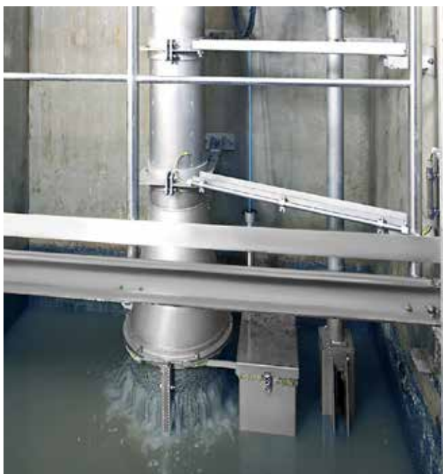
Wastewater pre-screening in the intake structure with a HUBER Pumping Stations Screen ROTAMAT® RoK4.
