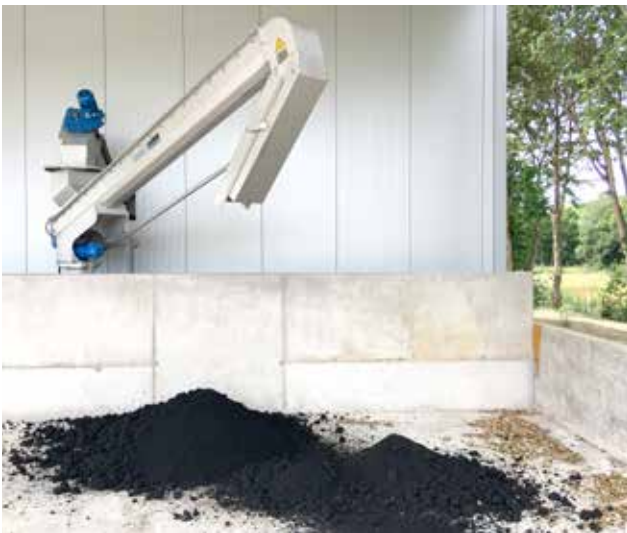
Collision protection in front of the HUBER Screw Conveyor Ro8 TC.
