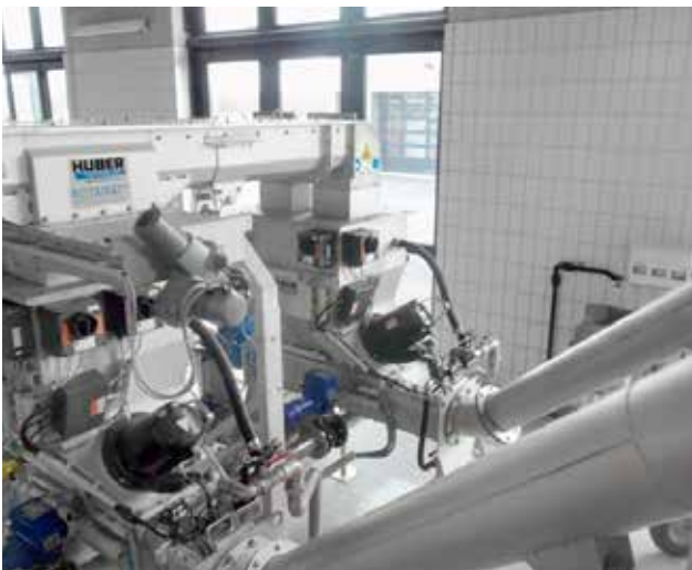
Intermediate pusher for distributing untreated screenings to two HUBER Wash Presses WAP® SL.
