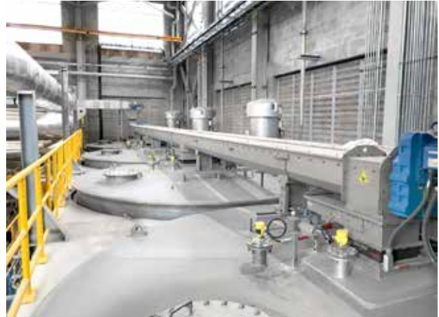
Horizontal transport of dried sewage sludge.
