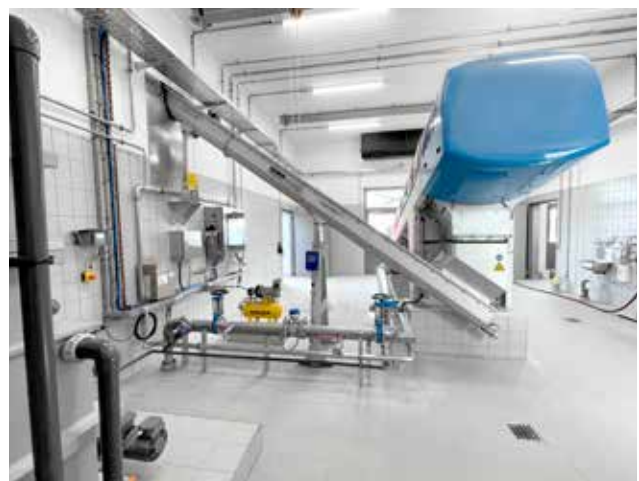
Inclined conveyor supply downstream of a HUBER Screw Press Q-PRESS®.
