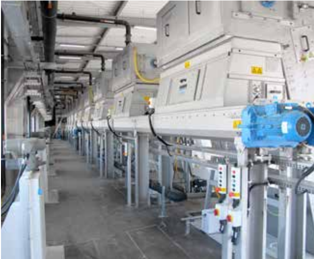
Redundant conveyor using a double trough diverter.
