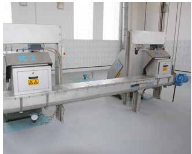
Two screens installed in parallel discharging into a screw conveyor.
