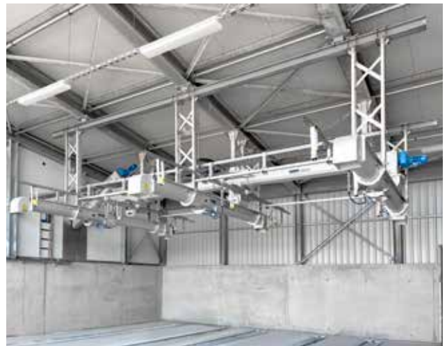
Ceiling-mounted distributor for disposal of dewatered sludge in containers.
