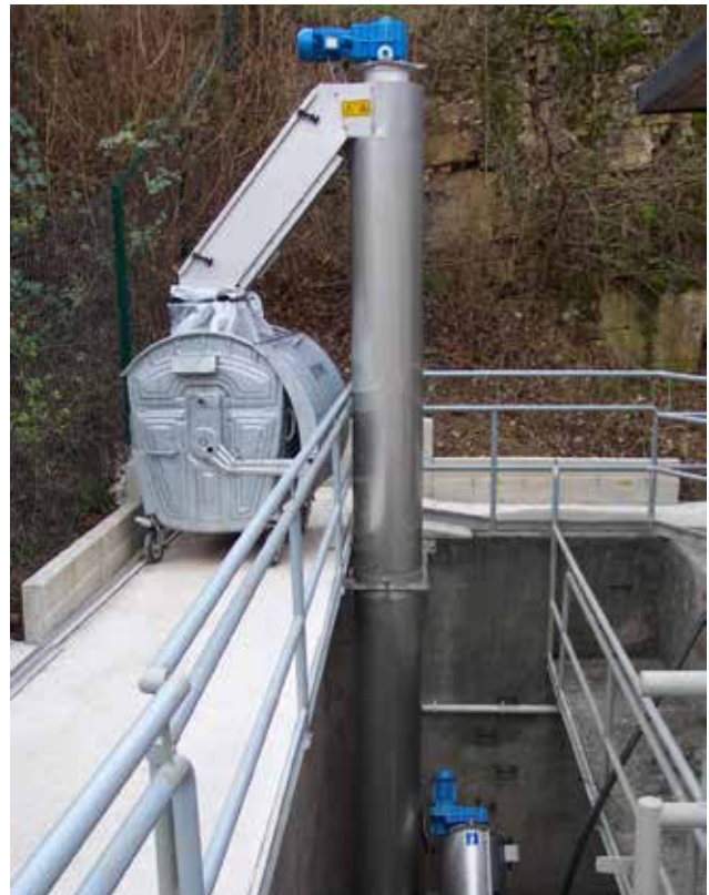
Vertical discharge of screenings from a micro strainer out of a deep manhole.
