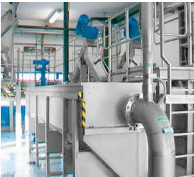
Above-ground redundant installation of a HUBER Longitudinal Grit Trap ROTAMAT® Ro6.
