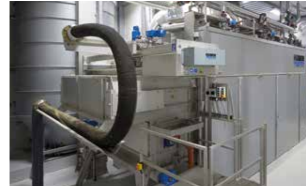
Sludge feeding with HUBER extruder unit.
