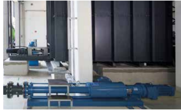
Sludge bunker and pump.
