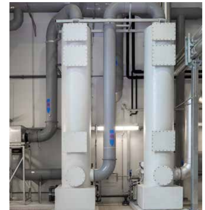
Two stage scrubber for odor control.
