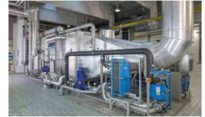
Condensation stage with heat extraction and fully automatic heat exchanger cleaning.
