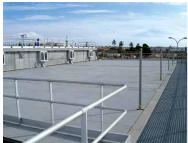
HUBER Sandfilter CONTIFLOW® 50 C, Rincon de Leon, Spain.
